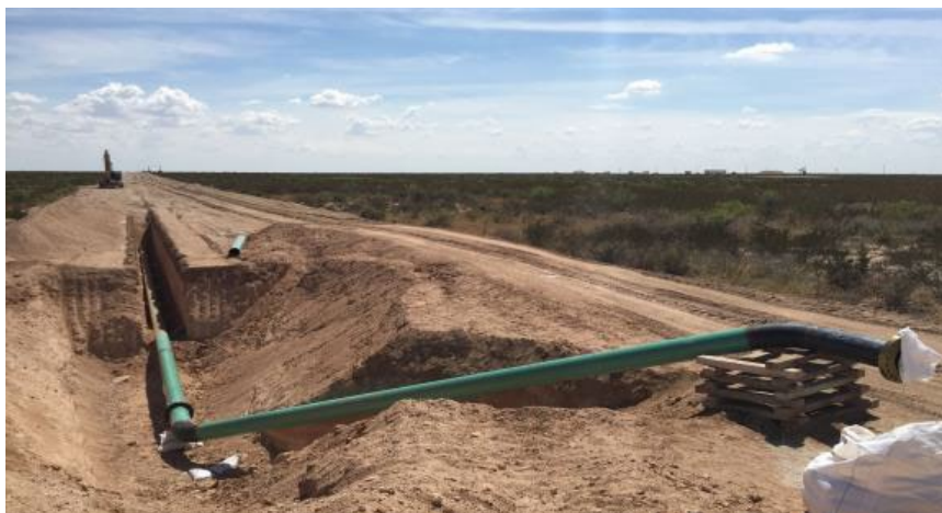
12", 24" and 30" Gathering Systems are also underway to tie in various regions of the Southern Delaware to the Caymus system.
